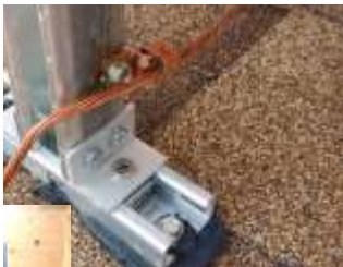
Example of a bad installation
